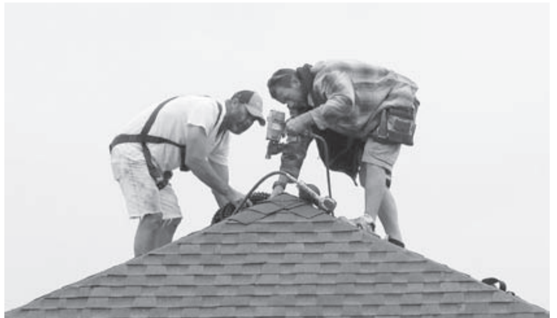
Roofers work on a new home in Panama City, Fla. The Federal Reserve released its Beige Book report on Wednesday, April 15, 2015. (Andrew Wardlow/News Herald via AP)
